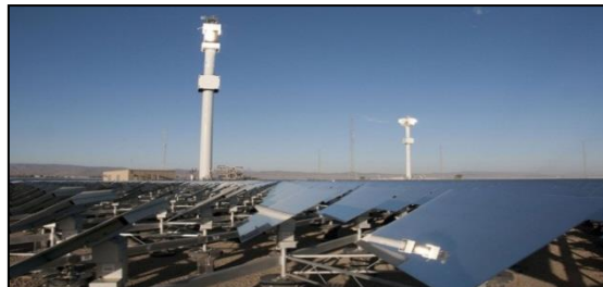
Fig 6: Solar power tower at Bikaner, Rajasthan, India
